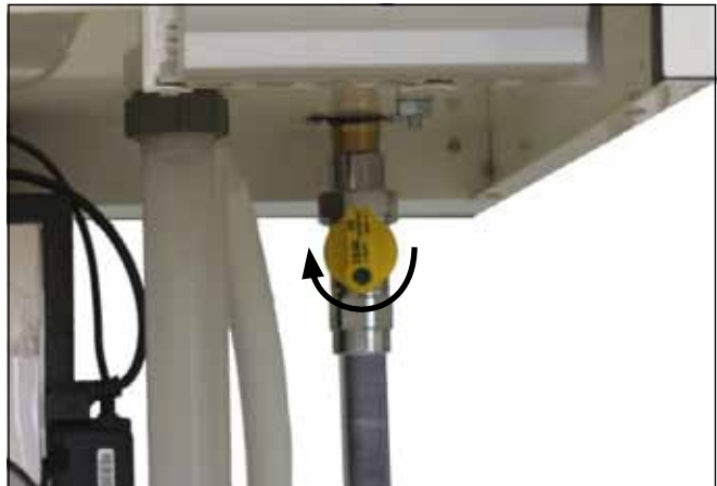
Figure: Gas connection
